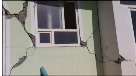
Fig. 1: Earthquake in Darbandixan (2017). (Source: Researcher)
